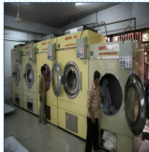
Dryer at washing Section
