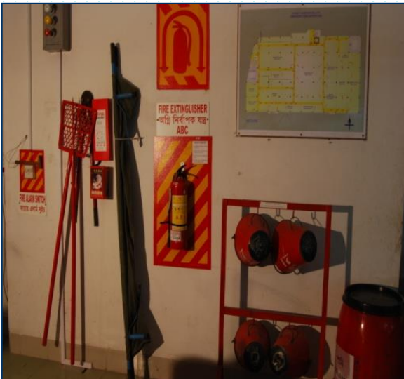
Fire Fighting equipment's
